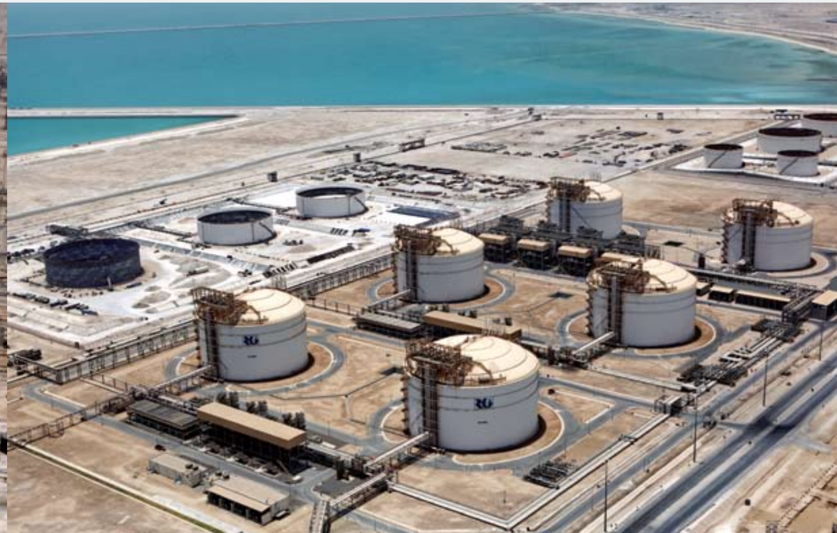
Aerial view of Common LPG Facility (CLPG)
